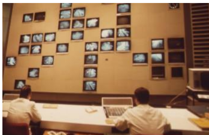
Figure 2-1 Example of an early CCTV system (taken from [10])
